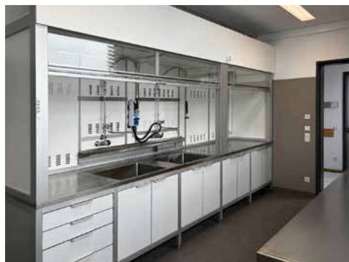
The new extraction system for breathing apparatus workshops sets new standards.
