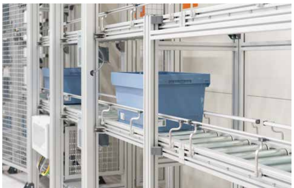
The PLC also handles the intelligent buffering of orders for which materials have been picked in more than one box.
